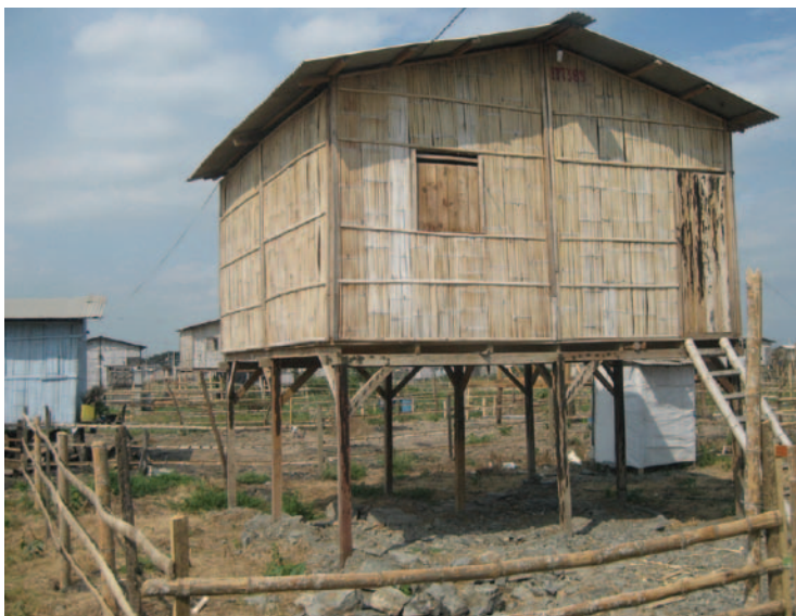
Families in San Bernabe prepare for the rainy season and construct their houses on stilts.
